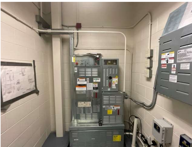
29 - ELEVATOR CONTROL ROOM
