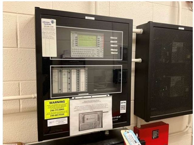
28 - FIRE ALARM PANEL
