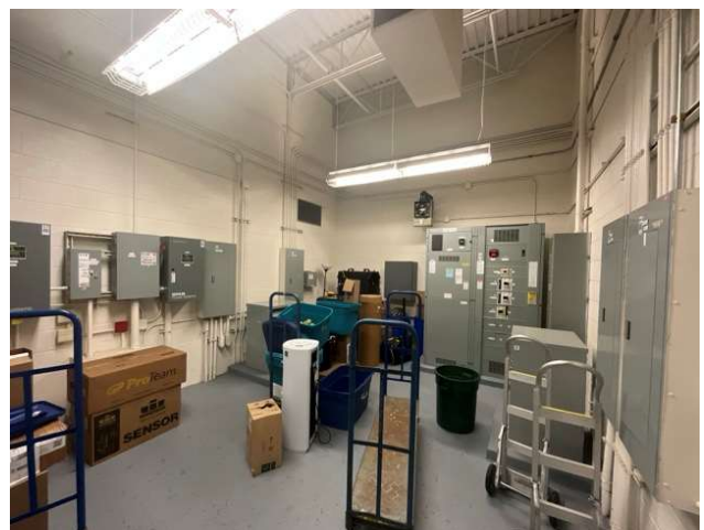
24 - MAIN ELECTRICAL ROOM
