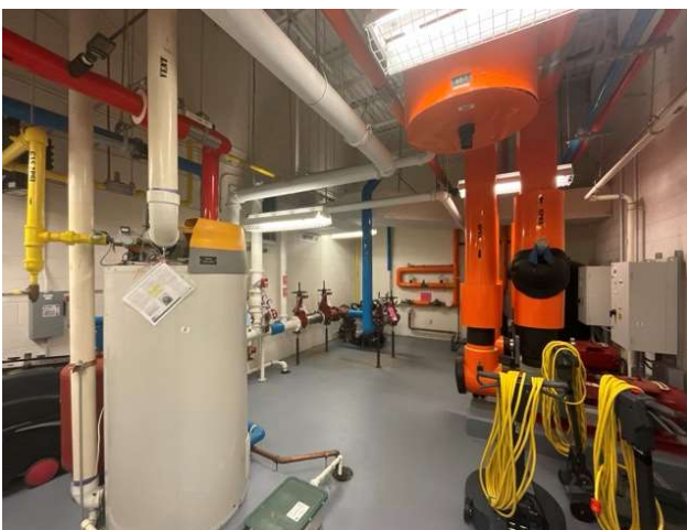
23 - MAIN MECHANICAL ROOM
