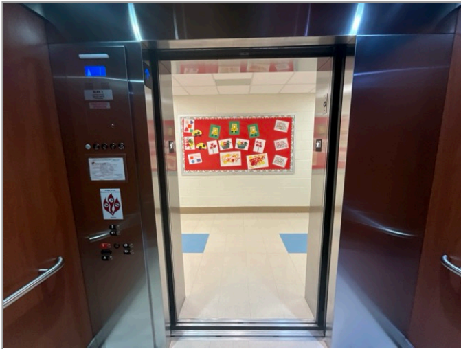
LOBBY LOOKING AT CAB
